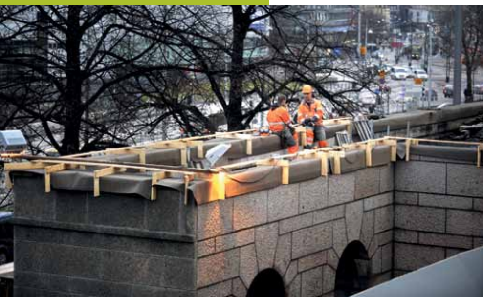
A new accessible entrance is being built in the old housing wing, along with facilities for visitor services.
